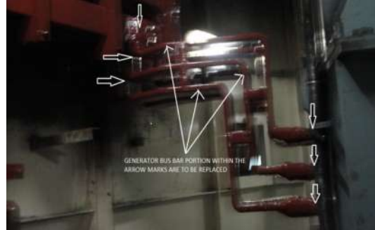
Position of the Generator terminal lead bar to be replaced
